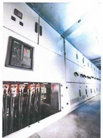
Today, Eaton's xEnergy can provide as much as 5,000 A via a single feeder section
